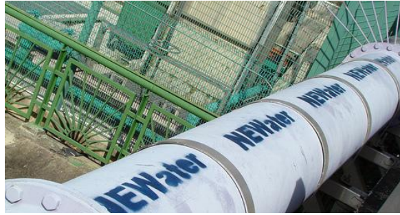
A NEWater Pipeline in one of the 4 NEWater plants Obtained and reproduced with permission from Flickr – xcode
