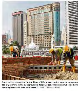
Construction is ongoing for the River of Life project, which aims to rejuvenate the city's river. In the background is Masjid Jamek, which is being restored with its original tiles. PHOTO: ARCHITECTURE/HERALD, TRAVEL, LEONG
