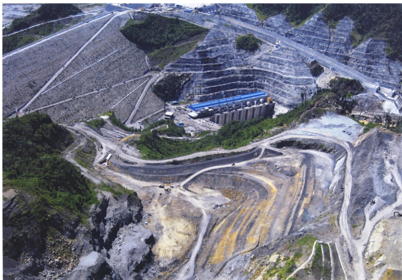
Fig. 1. An aerial view of the 2400 MW Bakun Hydroelectric Dam, under construction in 2010.
